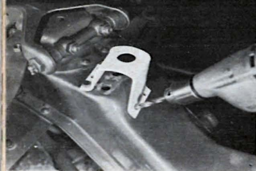
Special motormount supports, such as ones made by Hurst-Anco, can be installed by bolting or welding to frame.
