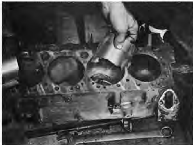
Stage one having been about completed, the cylinders have been almost completely removed. All that remain to go are the upper and lower decks.
