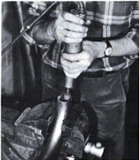
Before welding, you should grind out the inside of pipes and all rough edges.
