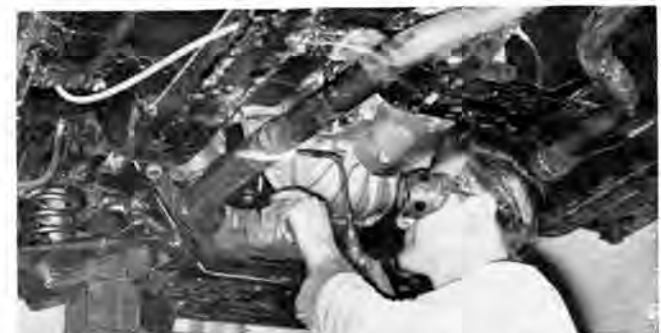
New section of head pipe is slipped over stock tubing and tack welded; then taken loose for finish welding. Left pipe is designed to allow oil filter to remain in original position.
