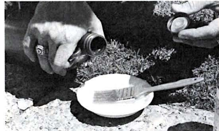
An industrial solvent should be used to clean and prepare the surfaces for the RTV primer. We used Toluene as it is recommended and it leaves very little residue. Alcohol, M.E.K., or Acetone could be used also.
